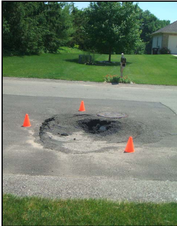
June 2009 Storm Damage
