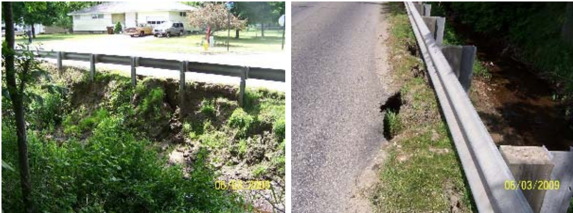
Drain bank erosion jeopardizing Riley Street
