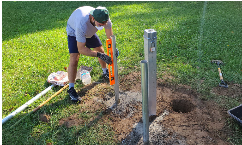
Former staff Land Use Planning Specialist James Kilborn installs well monitoring equipment at the Allendale water treatment facility. Right: A screenshot of the new Ottawa County Groundwater Reporter tool web page.
