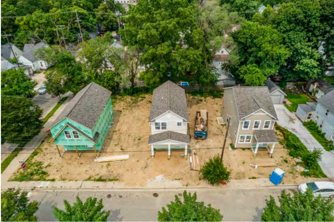
Construction on an ICCF Community Homes project in Grand Rapids' Baxter neighborhood in mid-2023. Credit: ICCF Community Homes
