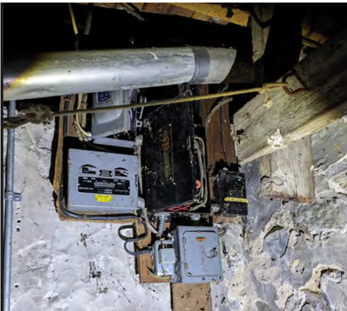
Existing Electrical Panel
