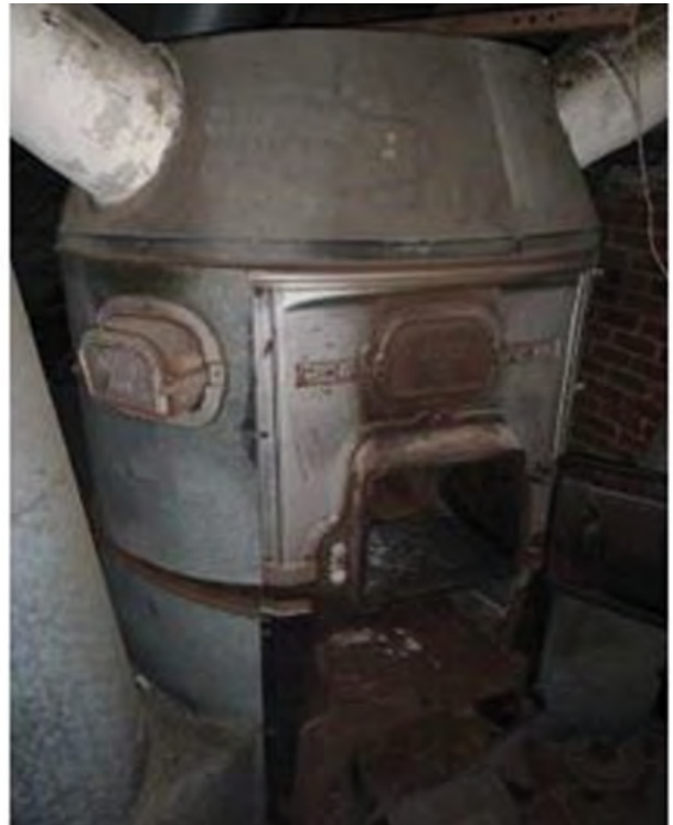
Existing Fuel Oil Furnace
