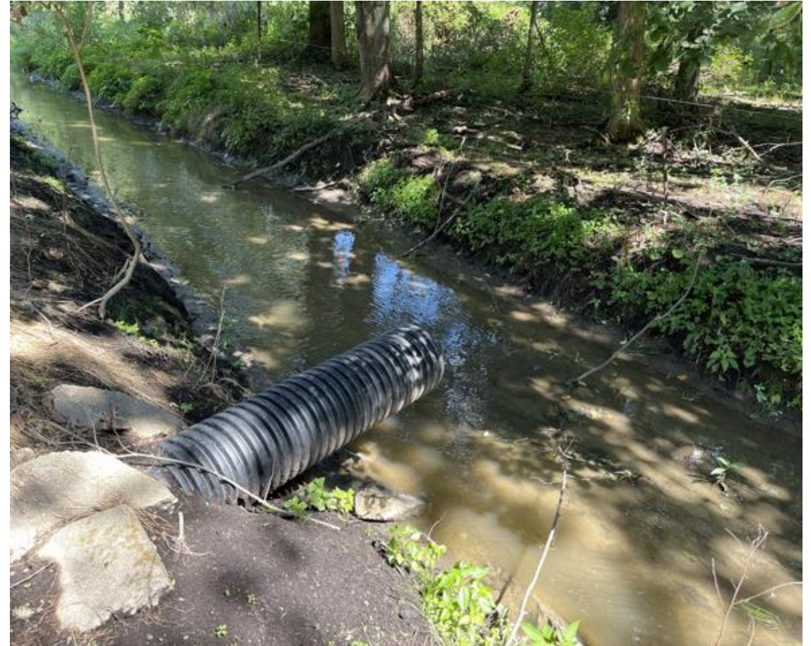
Tile Outlet, Station 12+40
