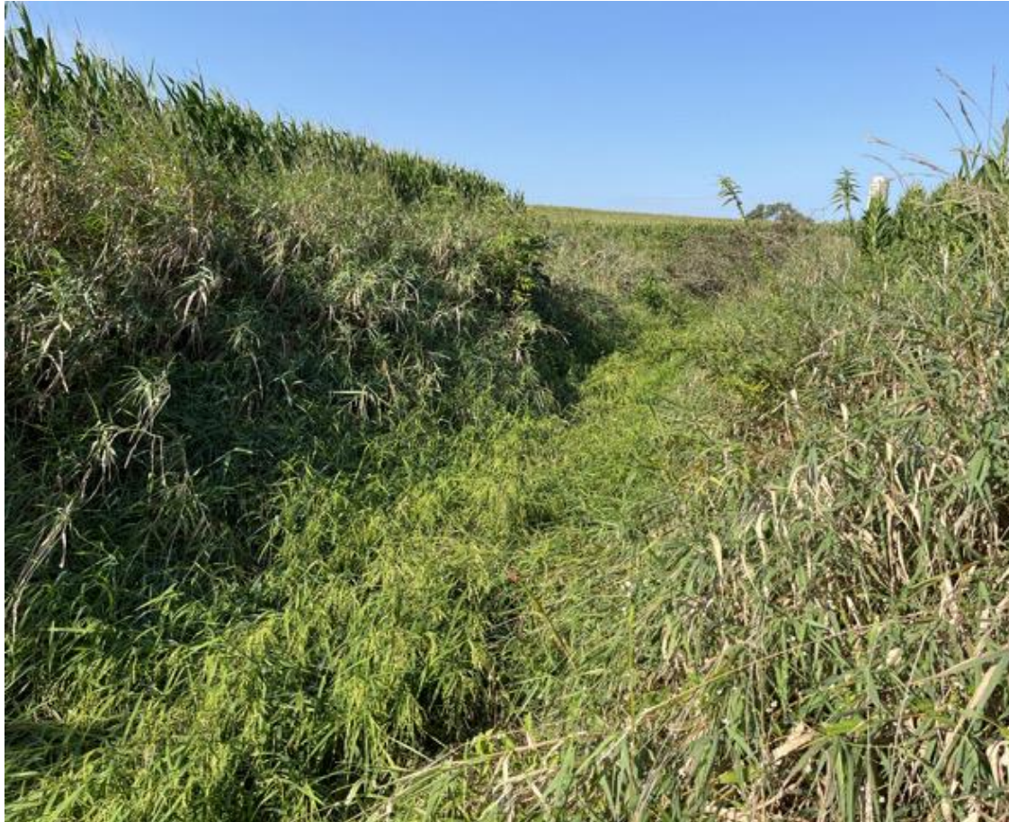
Vegetation Choked Channel at Sta 78+00
