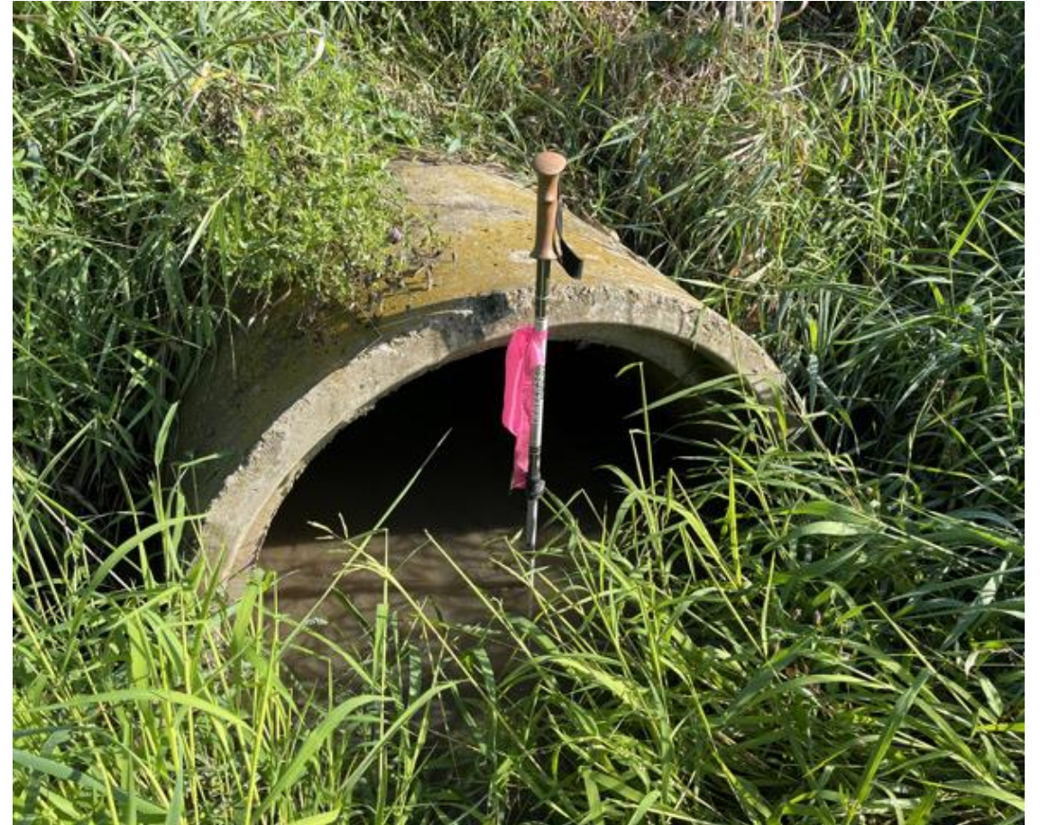
146 th St Culvert, partially submerged, 21" sediment depth
