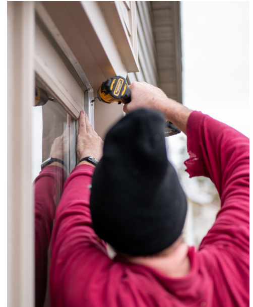
A contractor fixes a drafty door to prevent heat loss in the winter and heat gain in the summer.
