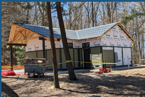
Restroom renovations include an addition of changing rooms and a new roof.
