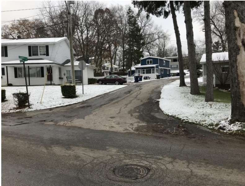
Lack of routine maintenance of existing leach basins
