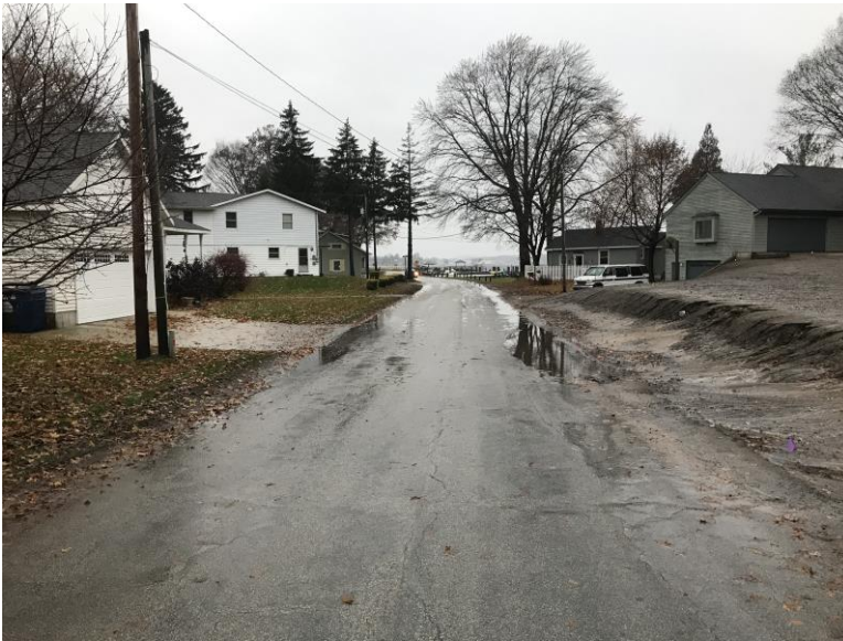
Standing water along both sides of Beach Dr west of Franklin Ave looking west
