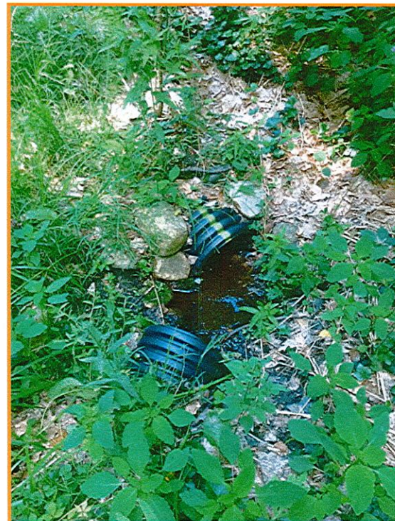
Left Photo: 12" RCP culvert inlet on north side of Lovell Road east of Spring Lake Road
