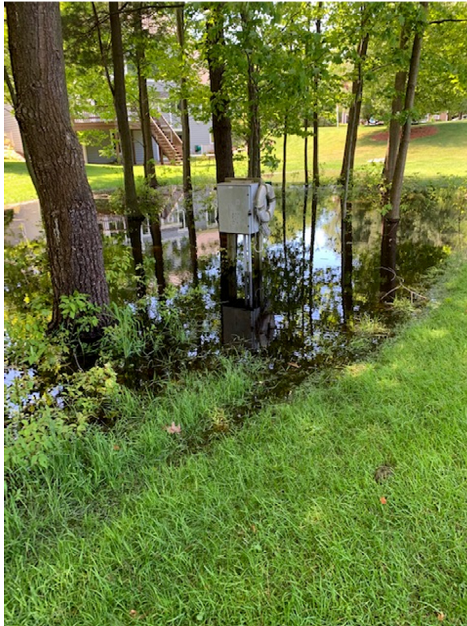
Retention Pond/Easement Area #5 – Ponding at back of 18823 Winnebago Drive (6/10/19)
