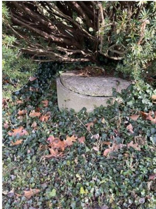
Manhole cover hidden under bush
