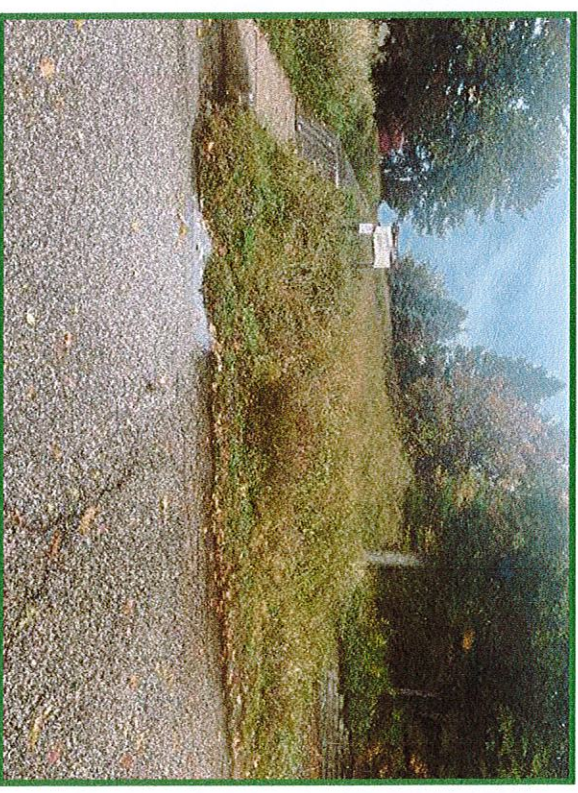
Ponding at Whispering Sands Drive and Sheldon Dunes Drive intersection.
