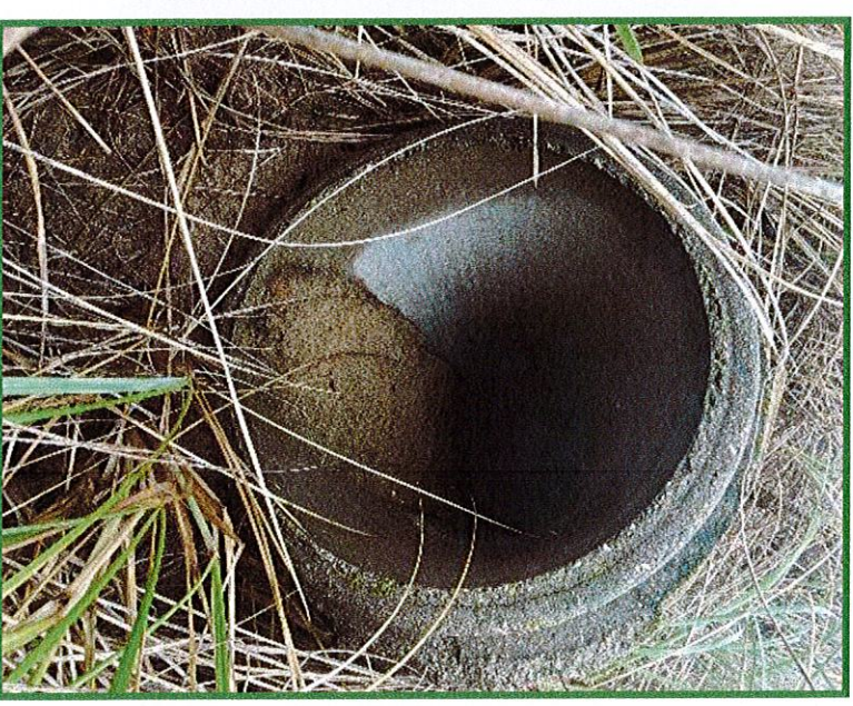
Sand in the pipe outlet immediately after rain event
