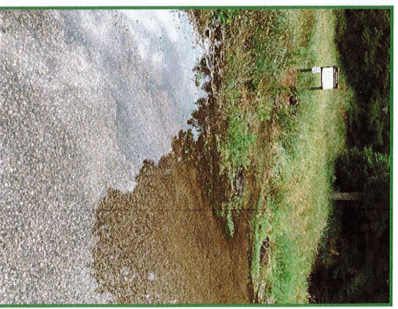
Standing water on west side of Whispering Sands Dr at public beach walkway.
