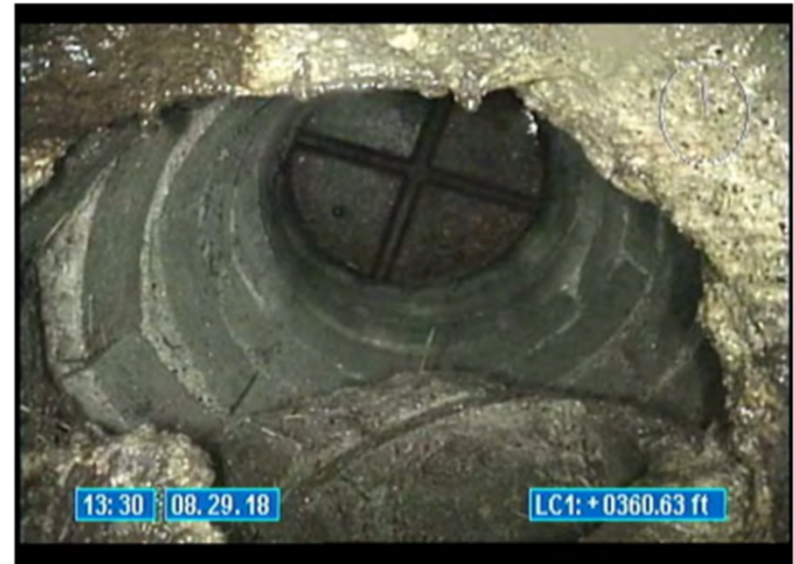
Block manhole structures are beginning to deteriorate.
