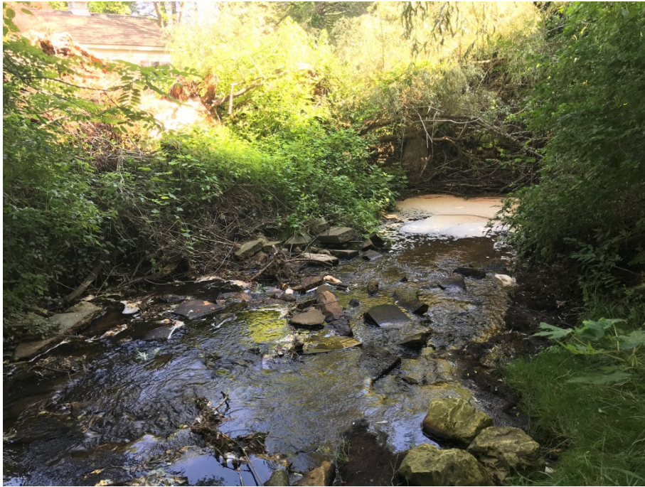
Debris (riprap) in drain and log jam downstream. Location is where school parking lot drains west towards Warber Drain.
