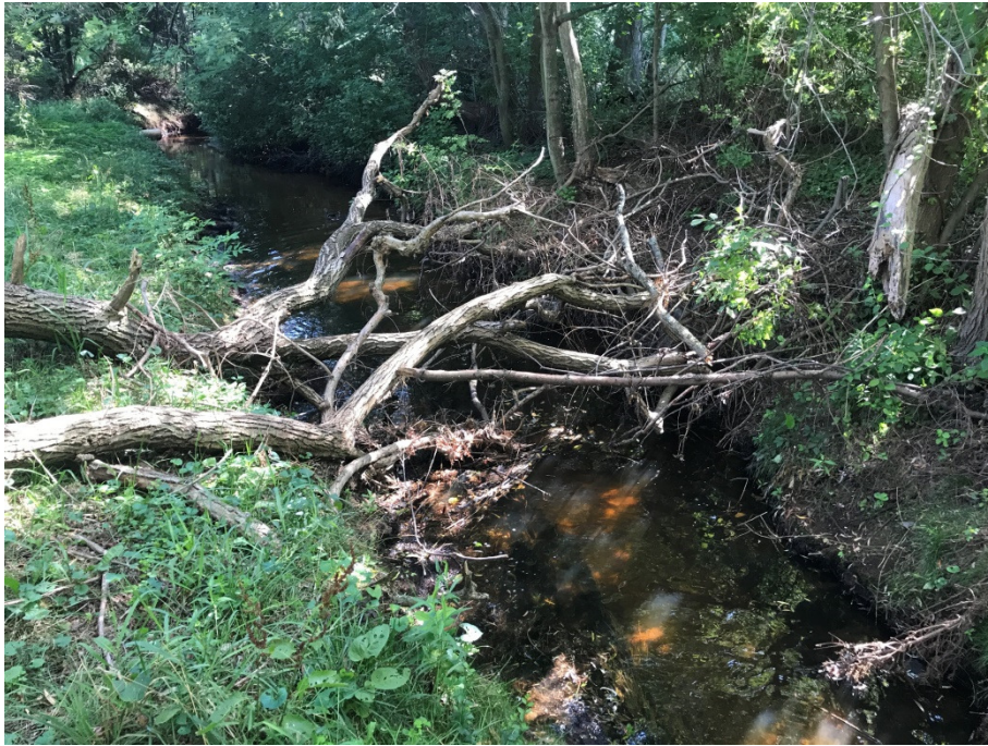
Log jam from fallen branches in river (see map). Branches appear to have fallen from willow tree on west bank.
