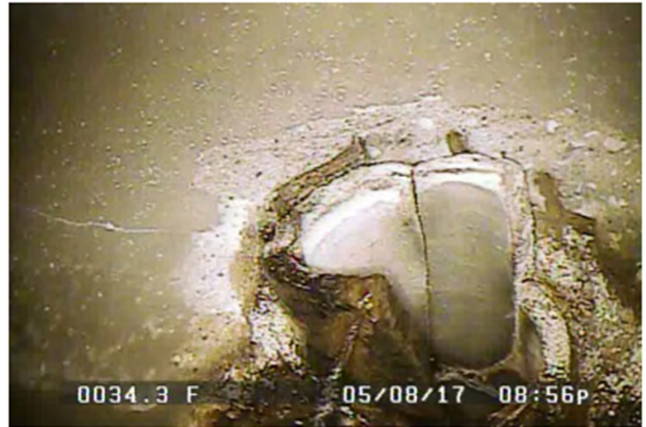
Cracked/Crushed/Collapsed Blind Taps are common in the Robbins Road Warber Drain storm sewer.
