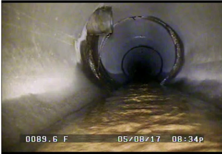
Protruding tap and mineral deposit buildup (encrustation) at joint.
