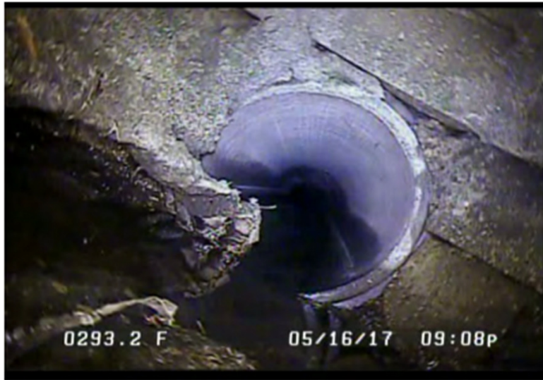
Mortar blocking inlet of pipe in manhole.
