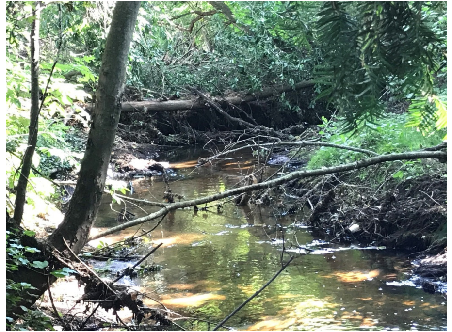
Fallen trees in drain near northwestern-most corner of parking lot
