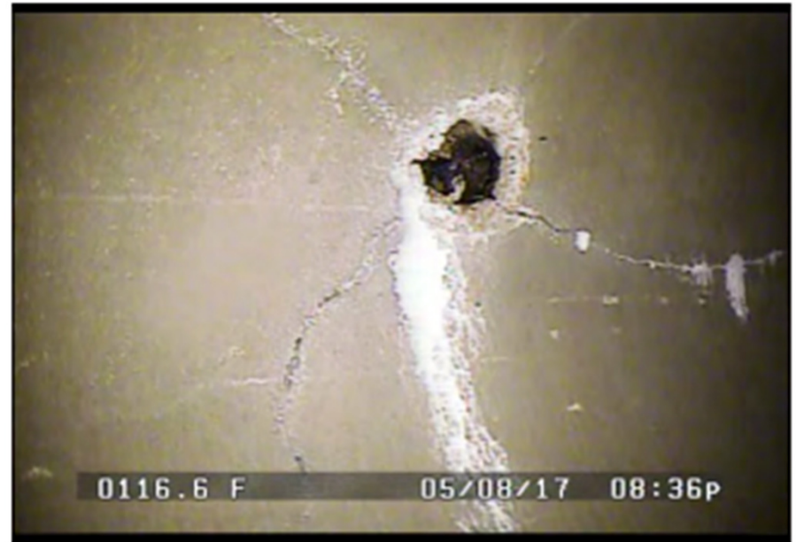
Cracking around lift hole of the 30 inch storm sewer.
