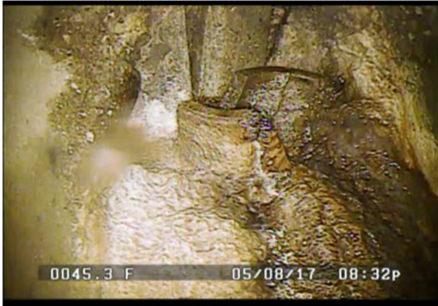
Collapsed protruding tap. These taps are located nearly entirely on the south side of the road and do not appear to have been properly sealed, and thus allow sediment to enter the storm sewer.
