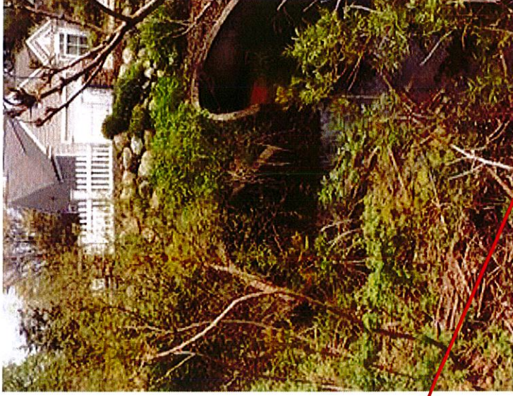
Overgrown trees and vegetation at the culvert south of Cobble field Lane.
