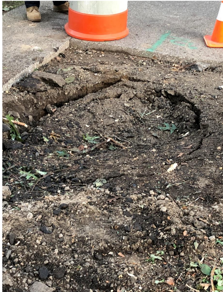
Sinkhole in Path (filled in multiple times and continues to exhibit signs of settling)
