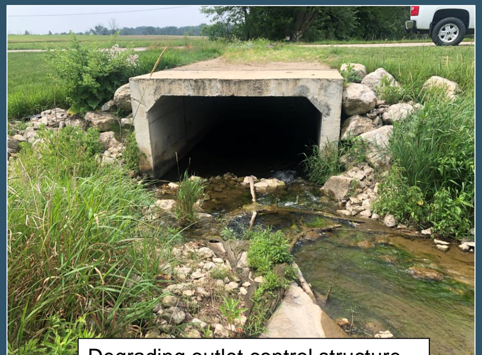
Degrading outlet control structure.
