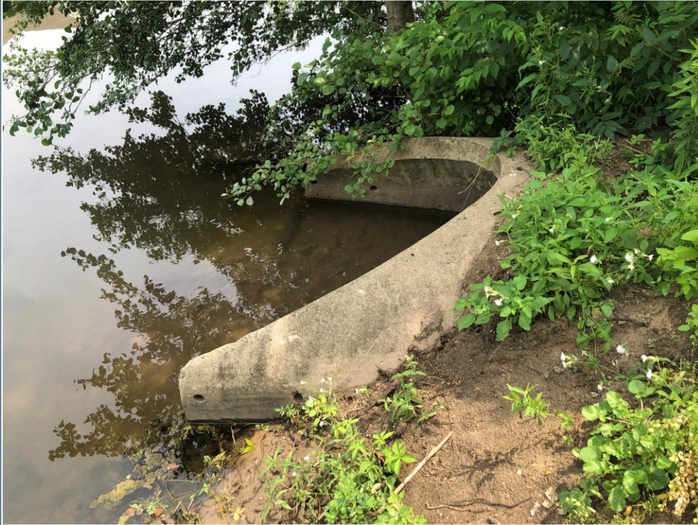
Undersized inlet culvert.
